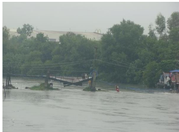
Tabon – Lambingan Bridge destroyed due to raging flood water
