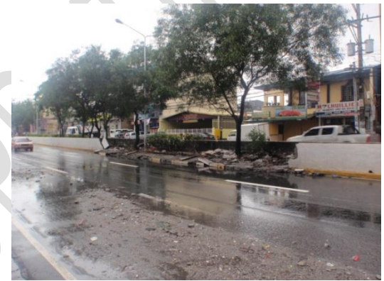
Concrete barrier destroyed as flood waters traverse this area
